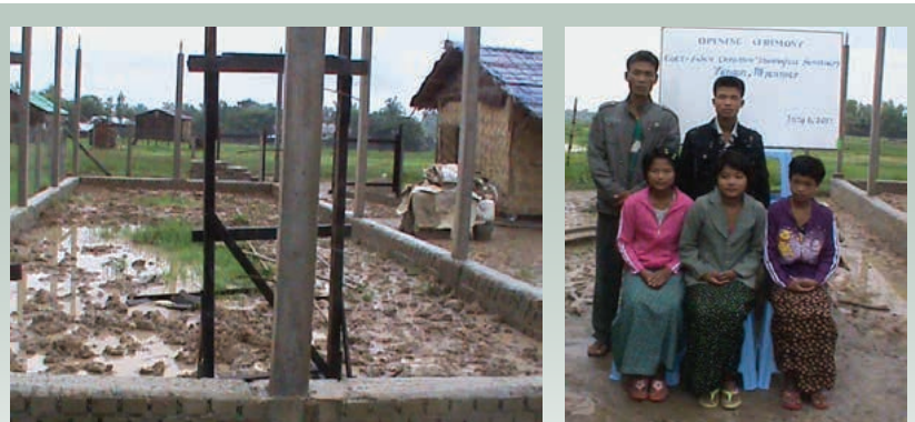
Ministry school starts in Myanmar: The new CoG7 conference here has enrolled its first class of five students. Supported by G. C. Missions, a new school building is under construction near Rangoon.
